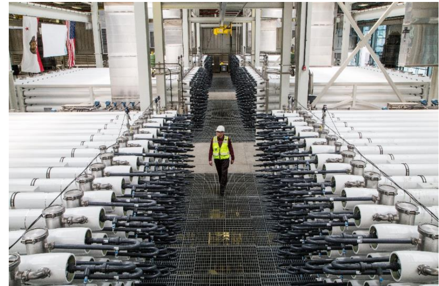
OCWD/OCSD – Groundwater Replenishment System
