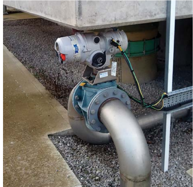
Figure 3 – Poor installation can breed poor maintenance. This control valve, installed underneath a raised tank, is not accessible for maintenance purposes.
