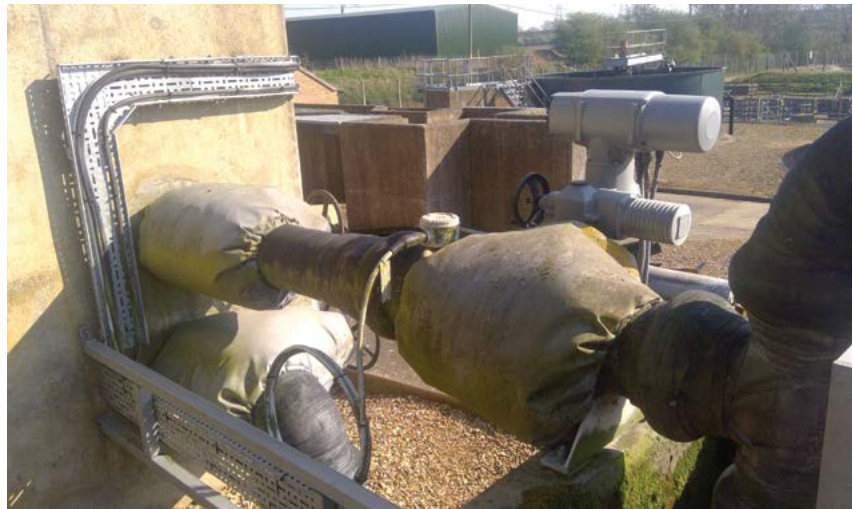
Figure 1 Poorly installed flow to full treatment flow meter.
