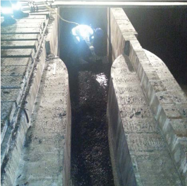
Figure 2: A large flume influenced by poor maintenance procedures allowing grit build up.
