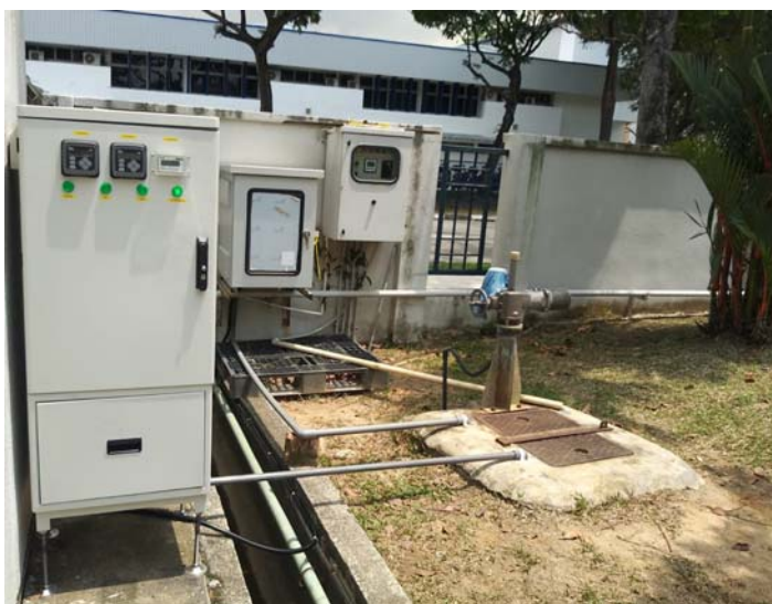
Figure 3.4 Image on setup of MES system at one of the industrial sites. (Source: EnvironSens Pte Ltd).
