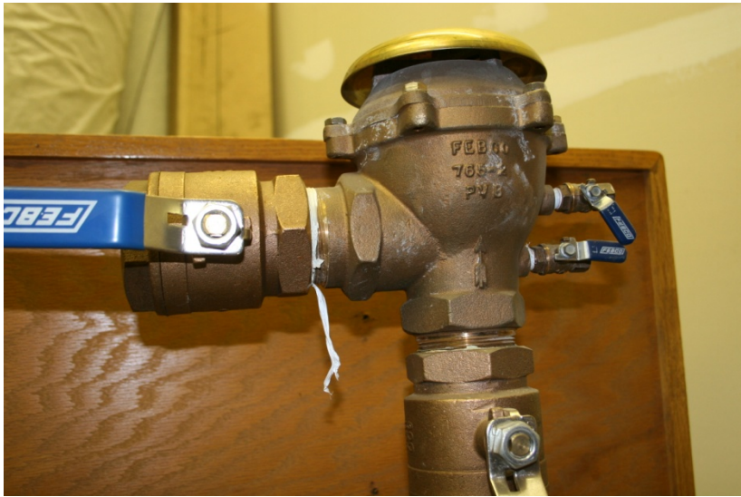
PRESSURE VACUUM BREAKER ASSEMBLY
