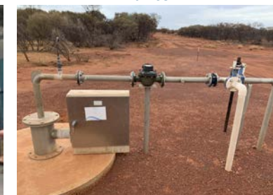
Sealed tanks and bores
