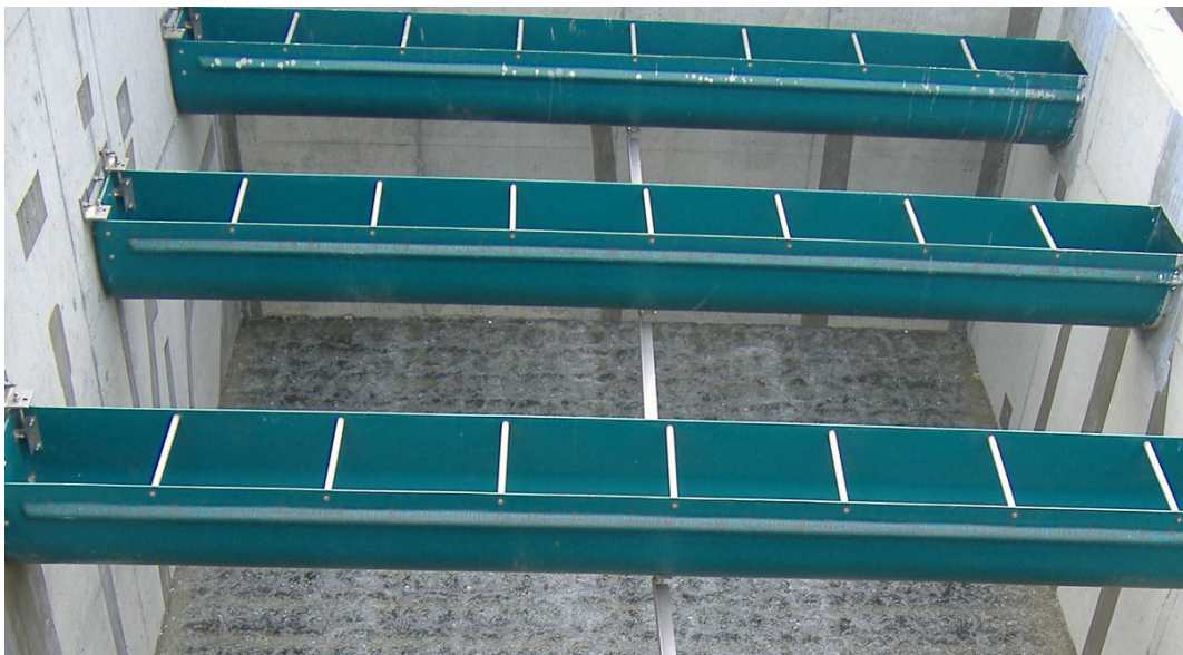
Figure 5.10: Example of used backwash water collection troughs.
