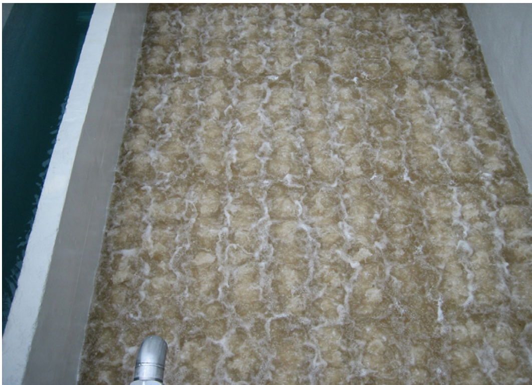
Figure 5.11: Example of a good backwash pattern.
