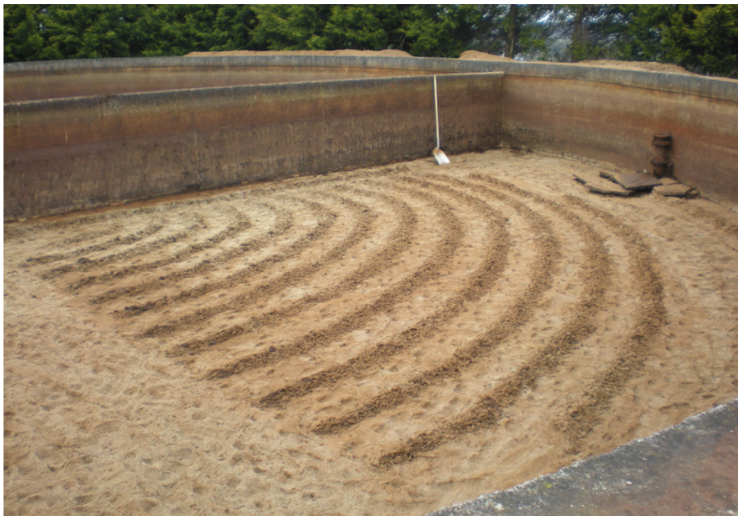
Figure 4.2: Example of a slow sand filter during cleaning/scraping.
