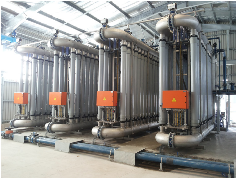
Figure 8.1: Example of an ultrafiltration plant.
