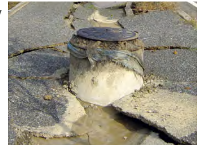
Manhole floats from liquefaction
