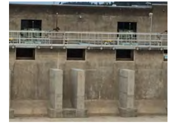
Basins, Reservoirs and Impoundments
