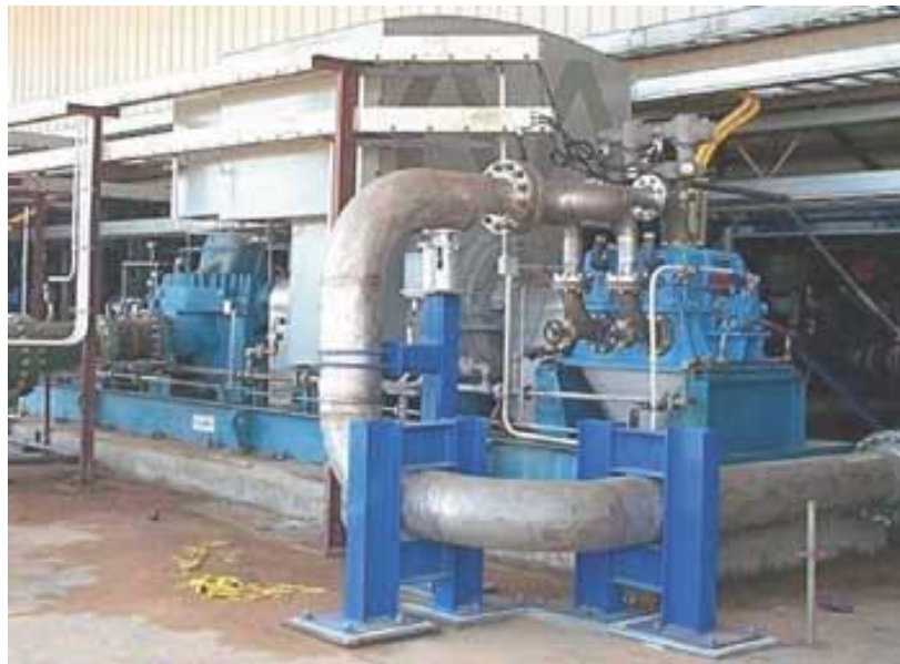
Figure 2-2: The Trinidad SWRO Plant Implementing Francis Turbine
