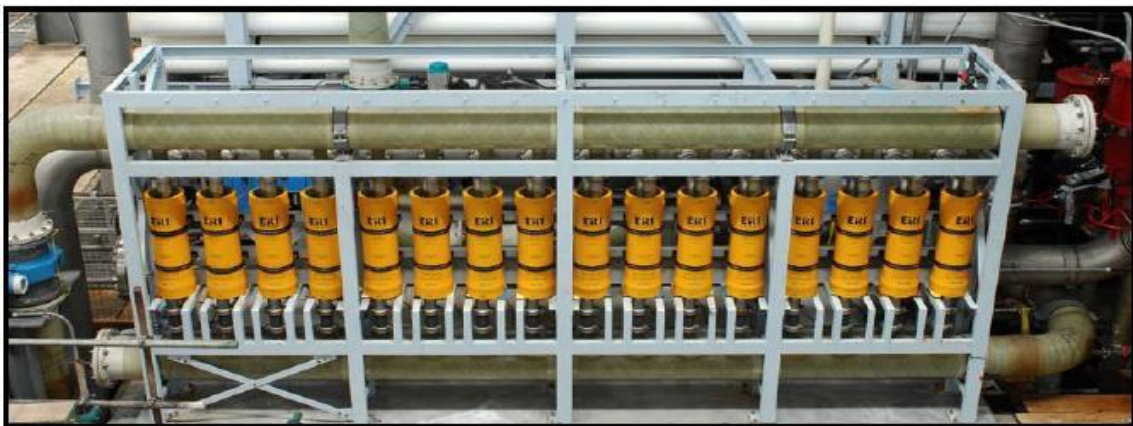
Figure 7-11: PX Device Array Serving SWRO Train 6A
