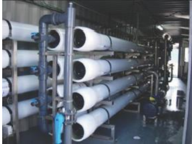
Figure 8-8: Desalitech CCD™ Unit
