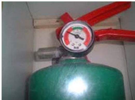
An empty fire extinguisher. Common in business settings. Bad news.
