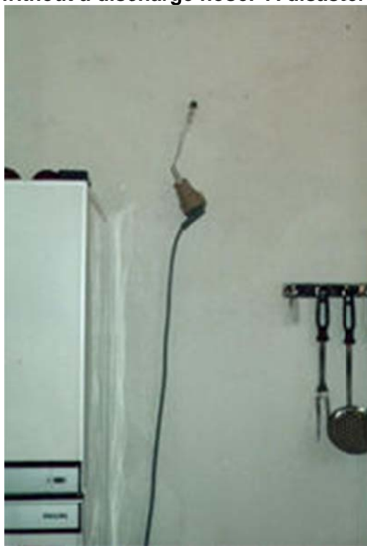
Dangerous Electrical Wiring. Fire waiting to happen.
