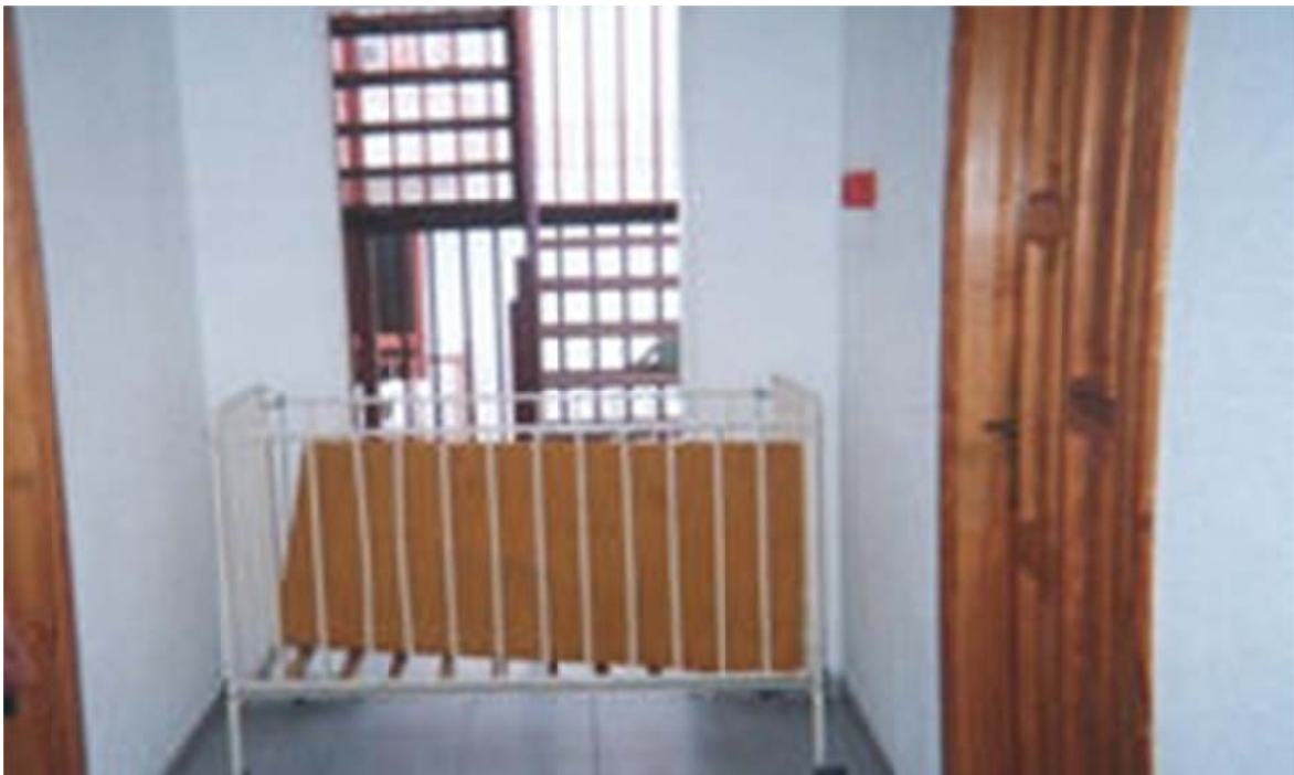
Blocked Fire Exit. Death trap.
