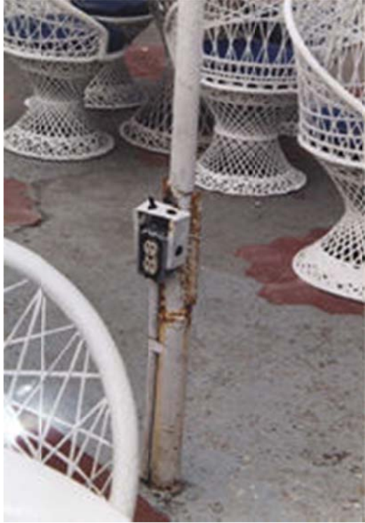
Dangerous Electrical Outlet
