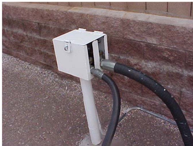
Propane Tanker truck hookup for mass storage facilities.
