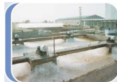
Effluent Treatment Plant
