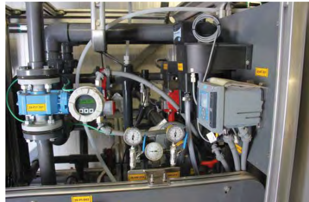
SUEZ Membrane Skid in WTP
