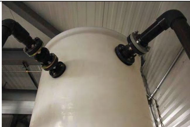
Flocculation Tank in WTP
