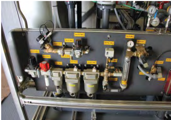
SUEZ Membrane Skid in WTP
