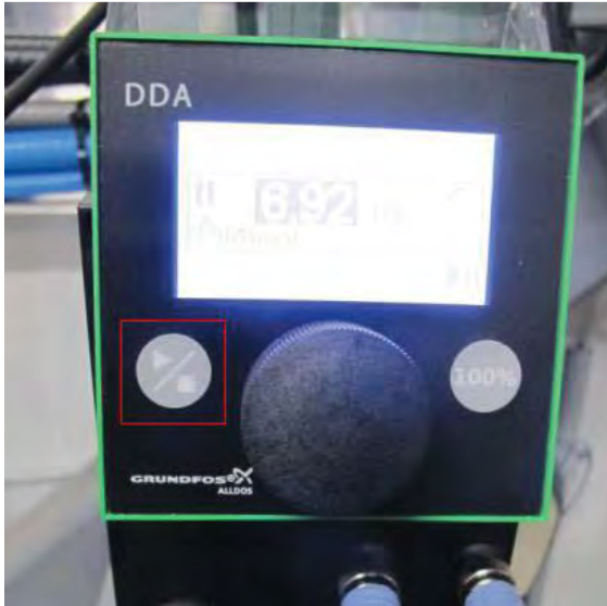
Figure 7. 7: Chemical Dosing Pump Start/Stop Button
