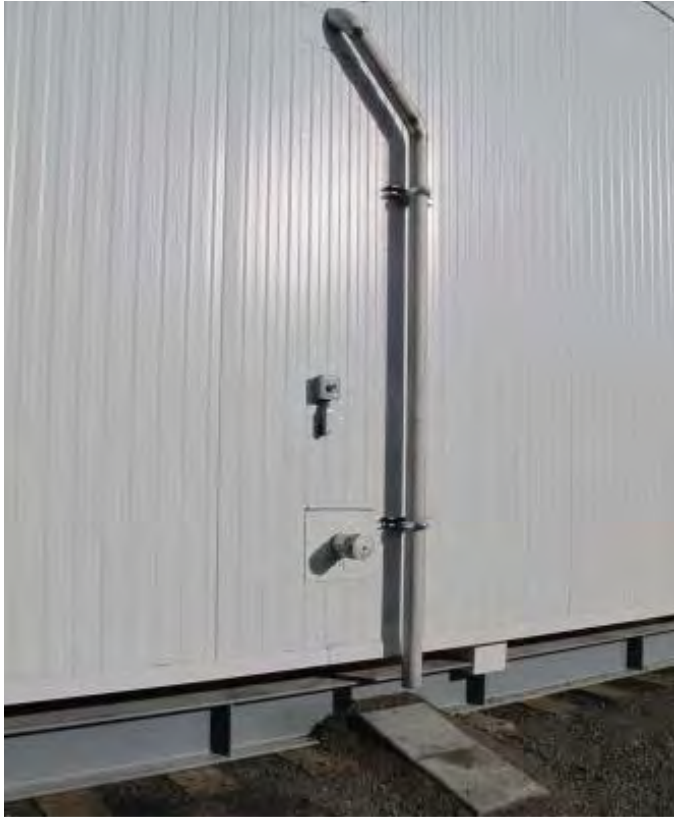
Figure 7. 13: Wastewater Tank Pump Out Emergency Stop Button
