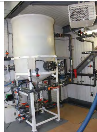
Flocculation Tank in WTP
