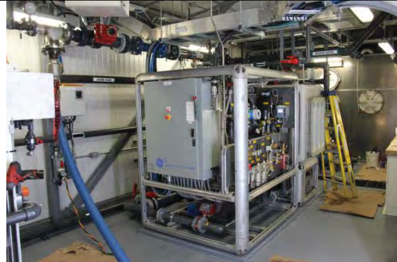
SUEZ Membrane Skid in WTP
