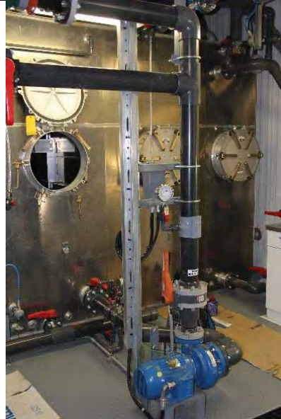
EQ Tank in WTP
