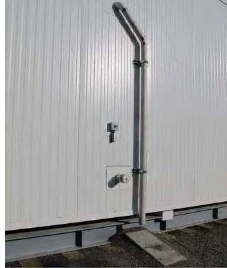
Wastewater Tank Connection (Outside)
