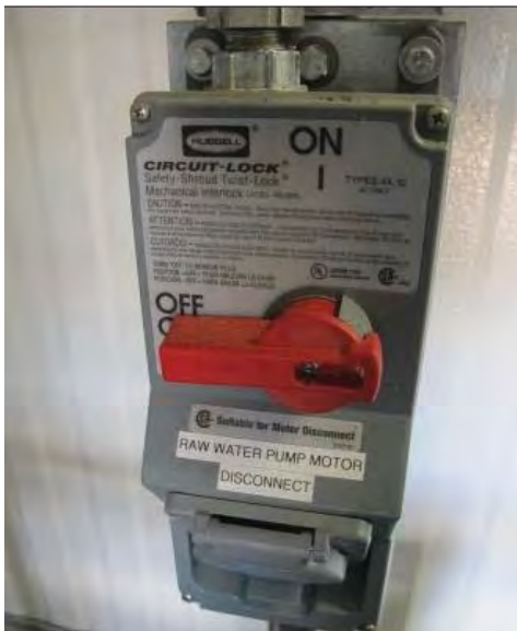
Figure 7. 4: Raw Water Pump Disconnect
