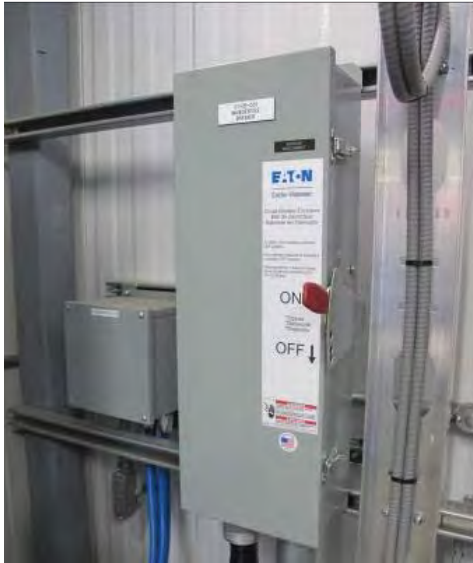
Figure 7. 3: Main Service Breaker
