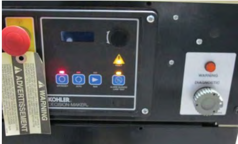
Figure 7. 11: Generator Emergency Shutdown Button
