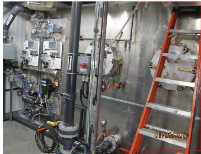
EQ Tank in WTP
