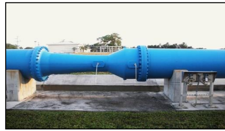
Figure 2 - 36-inch Venturi Meter
