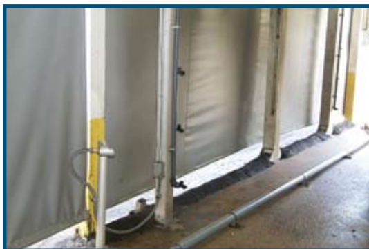
Figure 11. The gap between the overspray abatement curtains and the curb at this car wash facility allows wash water to escape outside the impervious area.
