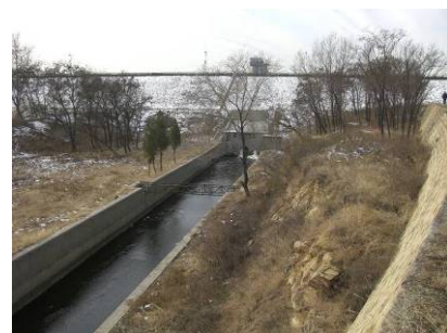
Maintenance flow discharge from Water utilization Dam ©CTII
