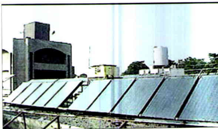
Figure 7.4: Flat-plate-collector-based solar desalination system installed at the Solar Energy Centre, Gual Pahari, Gurgaon
