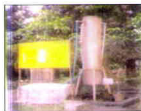
ARSENIC REMOVAL PLANT-OXIDE INDIA
