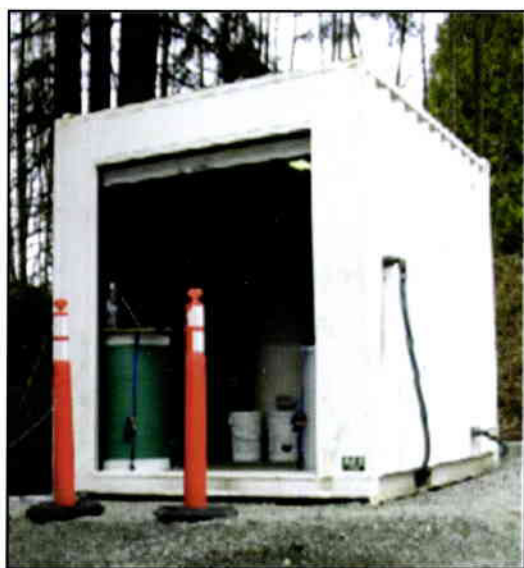
Figure 5.13: “IRON STOPPER” Containerized Treatment System, including the “DEFERUM™” hydroautomatic filter
