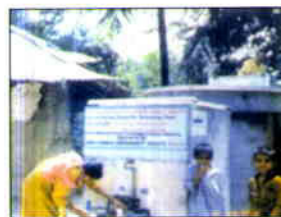
HANDPUMP ATTACHED ARSENIC REMOVAL PLANT-AIHH & PH
