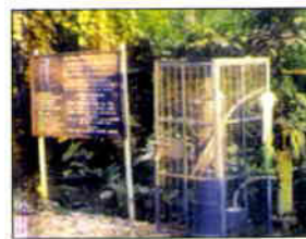
APYRON ARSENIC TREATMENT UNIT
