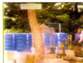
ARSENIC TREATMENT PLANT-PHED MODEL
