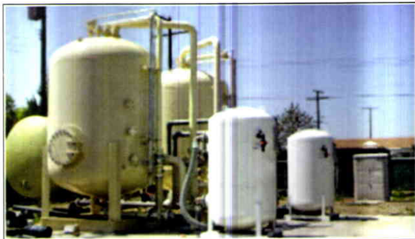
Figure 6.5: Siemens Nitrate Removal System
