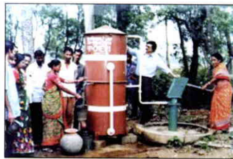
Figure 5.2: CMERI Iron Removal Plant
