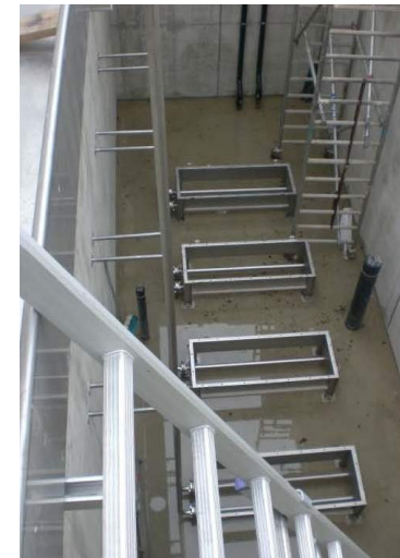
MBR filtration tank with air diffusers
