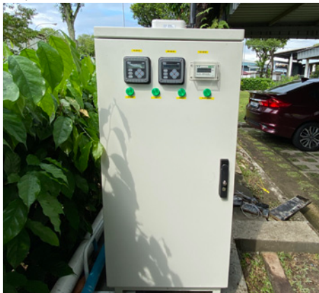
Figure 1. MES installed with IoT transmitter.
