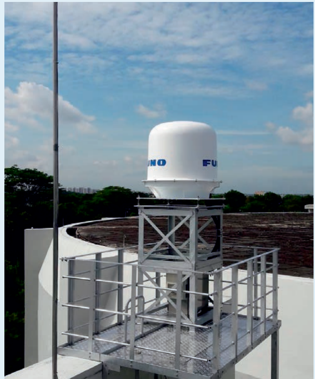
Figure 1: Picture of one radar installed at woodlands booster station
