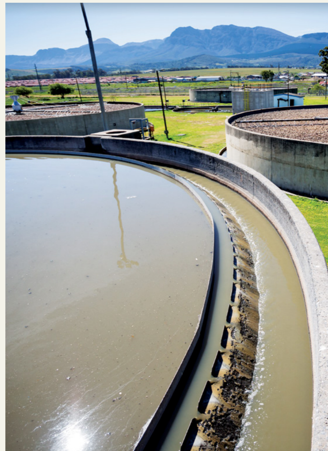
The Paarl Wastewater Treatment Works where good management standards are evident. This project is helping to improve biofilter efficiencies here. The biofilters utilise bacteria that feed on solid organic material and require oxygen for the biological oxidation process. “Through the WWF-Danish collaboration we realised that we needed a more consistent inflow over the stone beds (pictured here) where the bacteria live. When the flow is inconsistent, the bacteria die off, which, in turn, leads to a reduction in efficiency when the flow increases,” says Mark-Anthony Watson, senior superintendent: wastewater.
