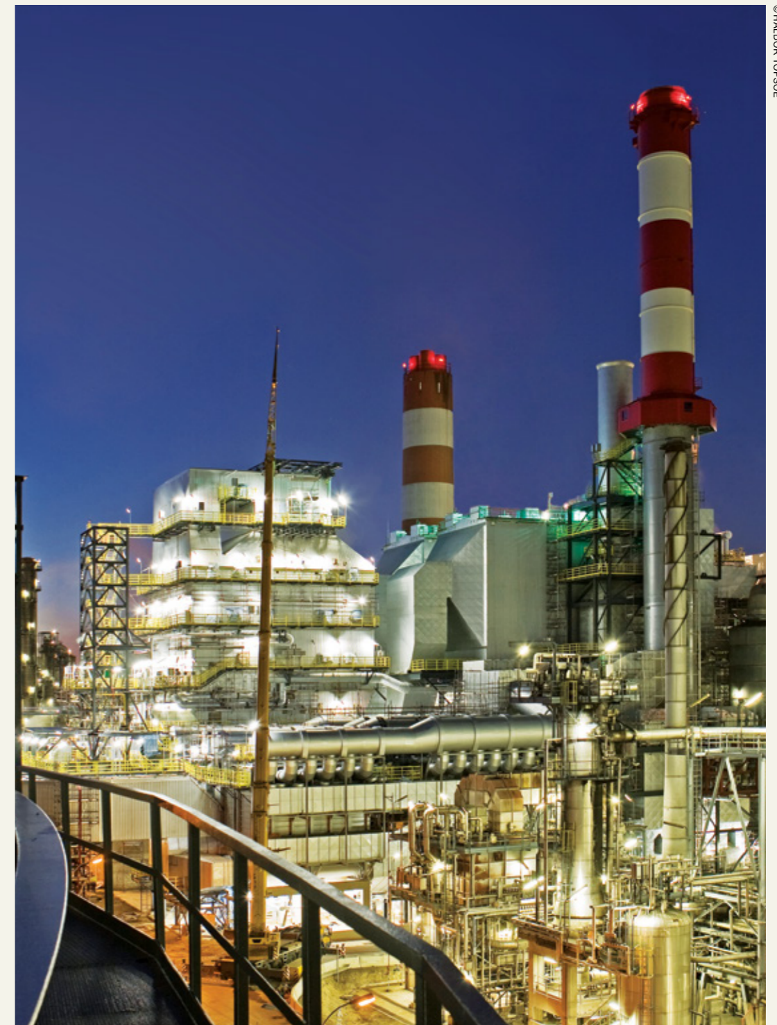
“SNOX™ technology is used in plants all over the world, including this plant in Austria. It is all about the correct technology for the process and this is what Haldor Topsoe is proposing for one of Eskom’s largest power stations, Majuba, in South Africa’s Mpumalanga province,” says Helge Rosenberg.
