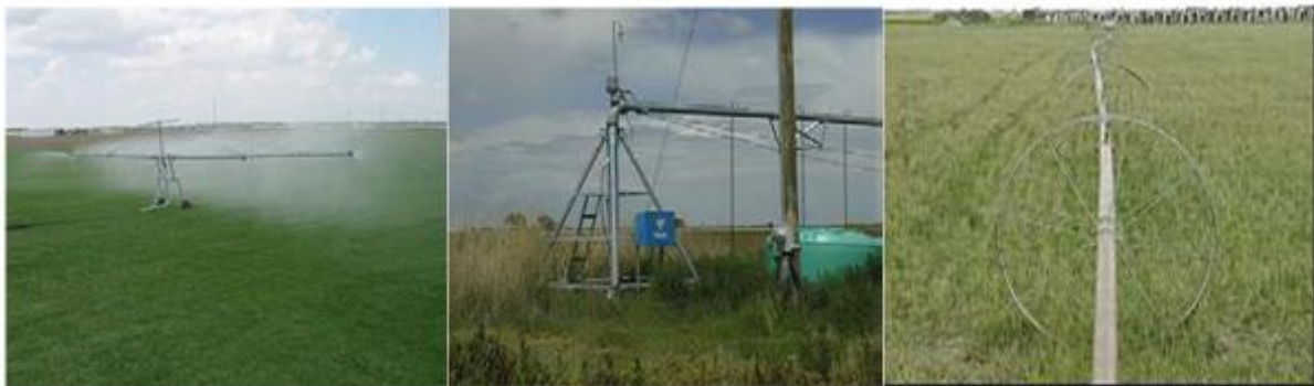
Fig. 36.1. Rotating type sprinkler irrigation systems.
