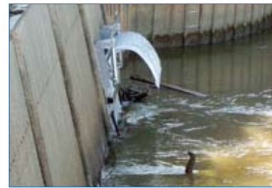
Fig. 5.2 a: Screen with automatic cleaning system
