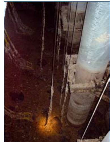
Fig. 5.3: Formation of a layer of scum in the pump sump
