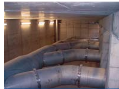
Fig. 4.1.1.2 c: Integration of the individual discharge lines in the direction of flow
