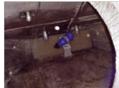
Fig. 5.7: Submersible motor mixer in a pump sump
