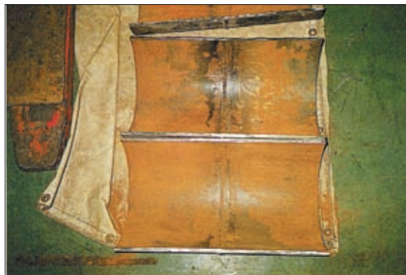
Photo 5.12 Inner surface condition of a carbon steel pipe treated with a nitrite based corrosion inhibitor during 15 years
