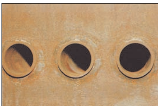
Photo 2.18 Inside of the boiler treated with a polymer based boiler compound during 1 year
