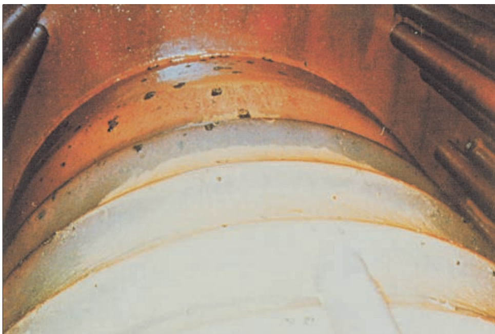
Photo 2.30 Corrosion of a boiler occurred during the stoppage
