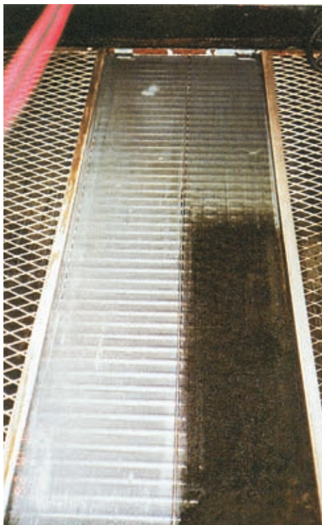
Photo 5.14 Effect of a chemical cleaning for aluminum fins Left side: after cleaning Right side: without cleaning
