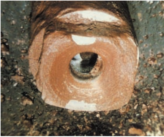
Photo 10.6 Scale of a spray nozzle under no chemical treatment
