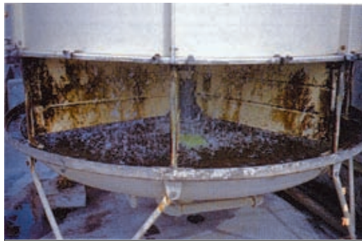
Photo 5.6 Algae adhesion to a cooling tower without chemical treatment
