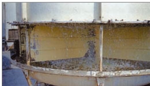
Photo 5.7 No algae adhesion to the cooling tower after using a tablet-type cooling water treatment agent
