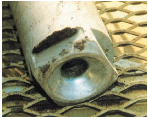
Photo 10.7 Clean spray nozzle treated with a scale inhibitor
