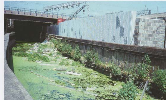
The concrete lined channel, choked with rubbish and green with algae, typified the degeneration of urban rivers when the photograph was taken, in the early 1990s. (The Lower Lea Project)
