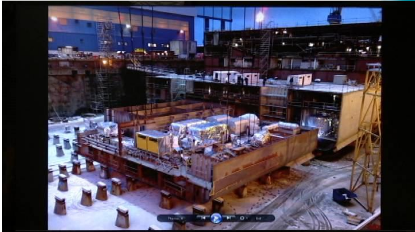
Floor Module with WWTP
