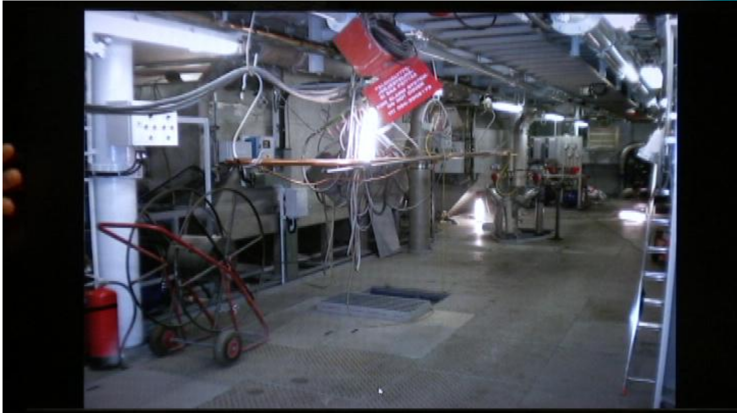
Complete MBBR System with DAF
