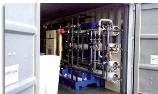
Aquamove™ MORO-16C comprises a SIRION™ Mega system with a dosing set and cartridge filters, housed in a 20' container.
