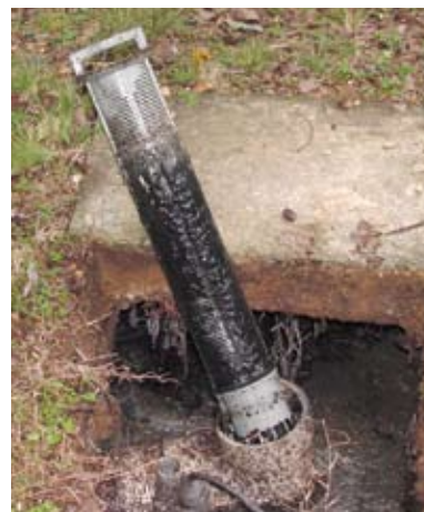
System inspections are a key component of management programs. Clogged septic tank effluent filters (above) can trigger calls for needed service, but regular inspections tailored to system type, setting, and use profile provide a better approach for ensuring long-term system performance.
