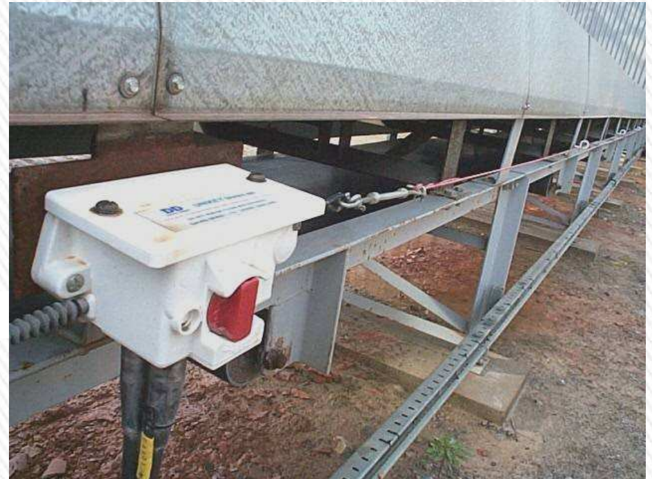
Safety Trip Wire
