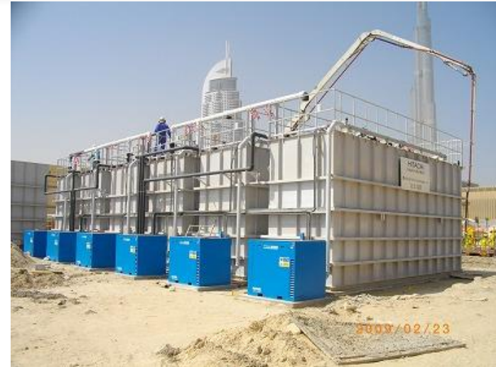
MBR TNK and BLOWER
