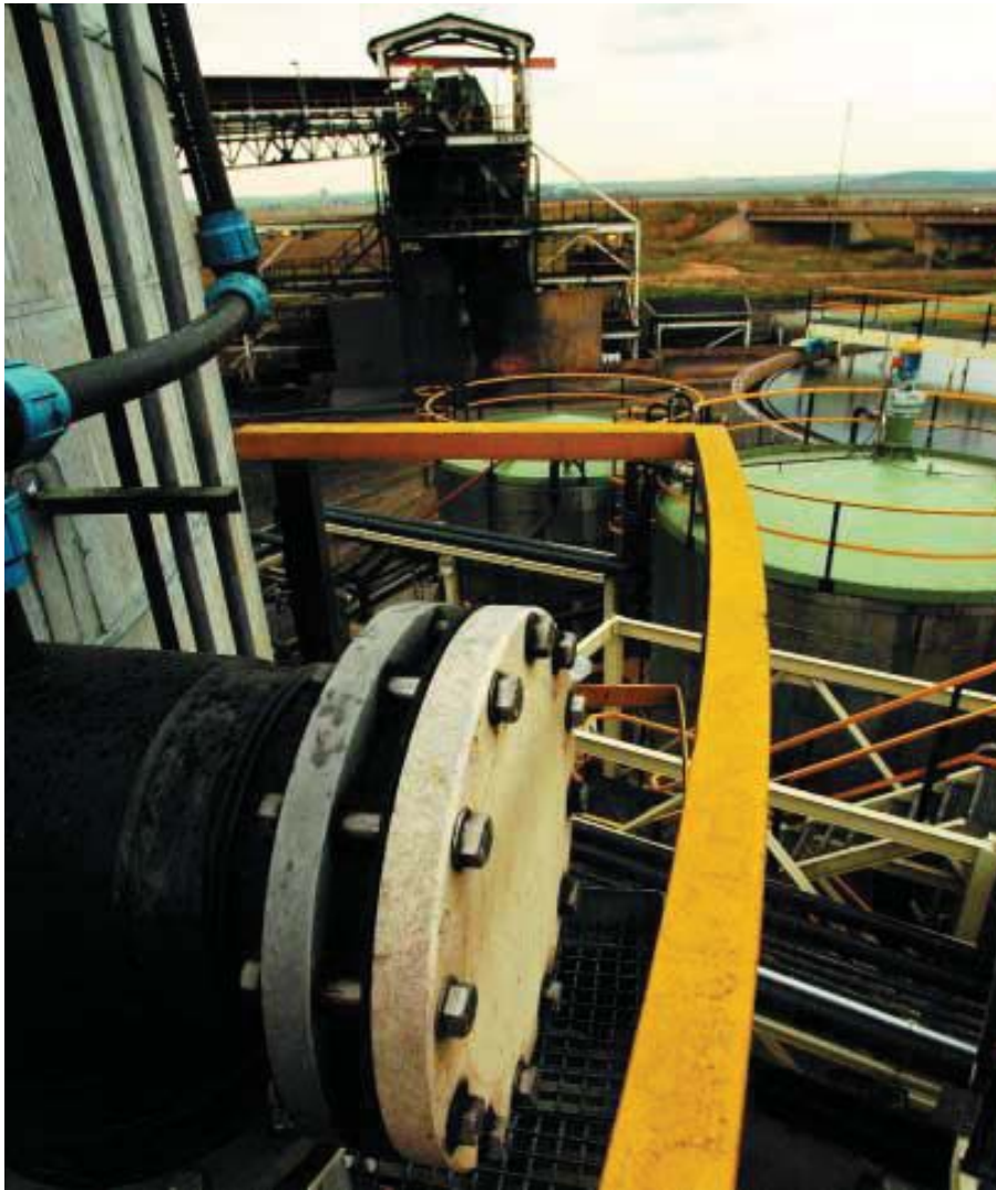
Figure 29: Biological water treatment plant at Landau Colliery
