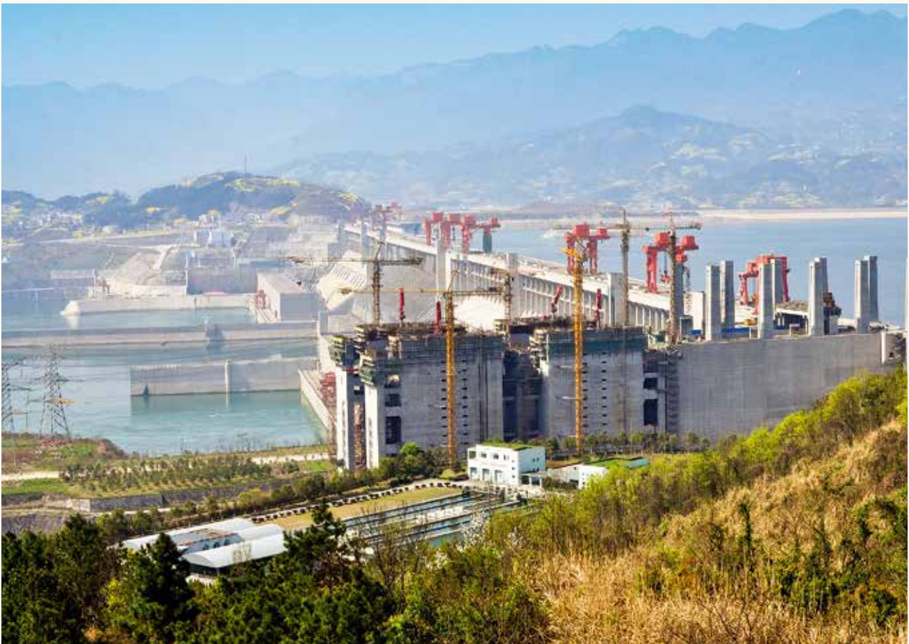
The Three Gorges Dam, spanning the Yangtze River in Hubei province, China, is the world's largest power station.
