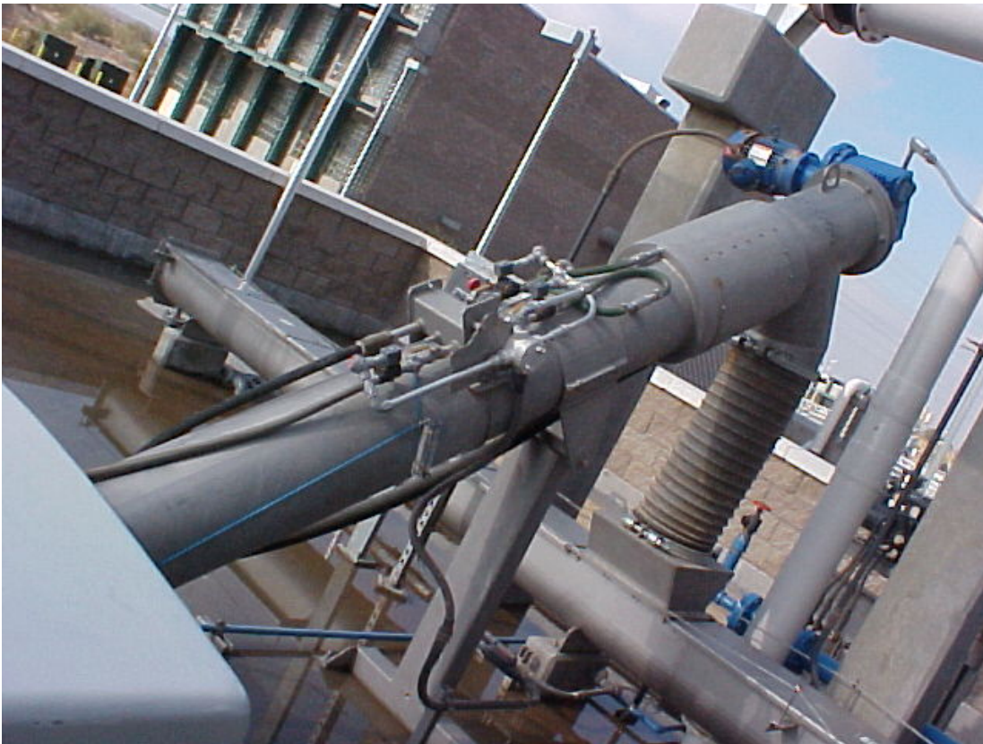
Rotating Bar Screens
