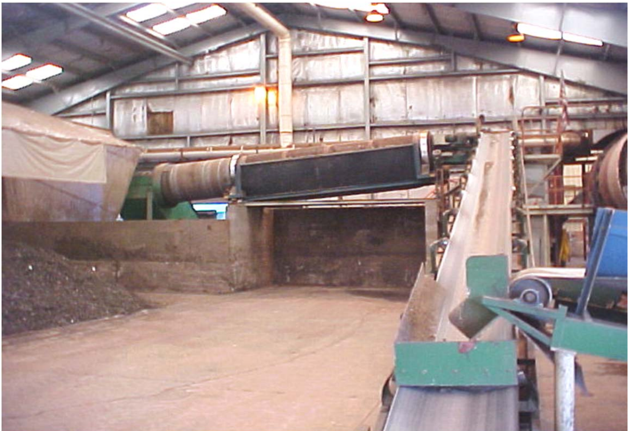
Example of a Sludge Press.
