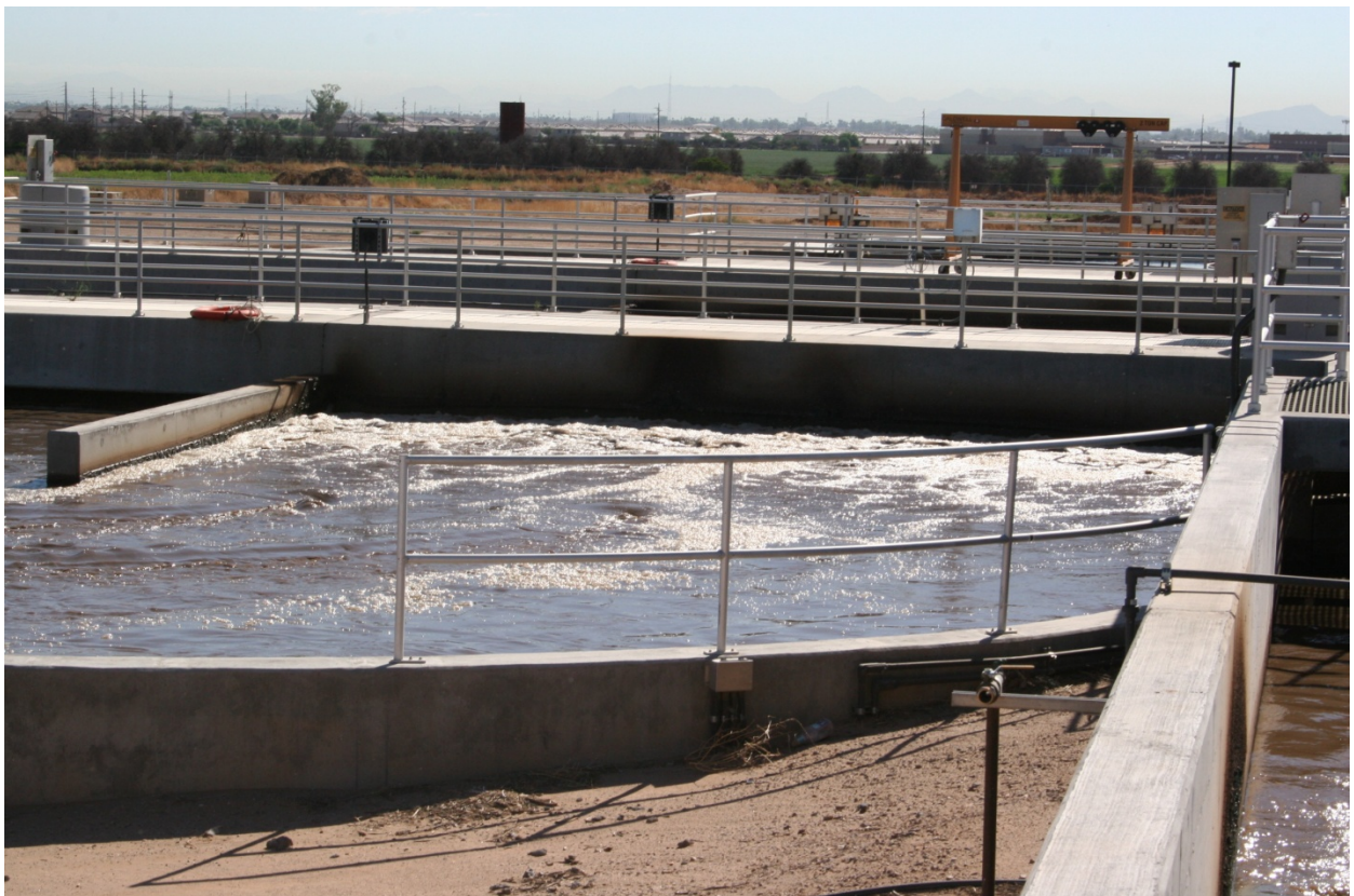
Oxidation ditches are used for nutrient removal.
