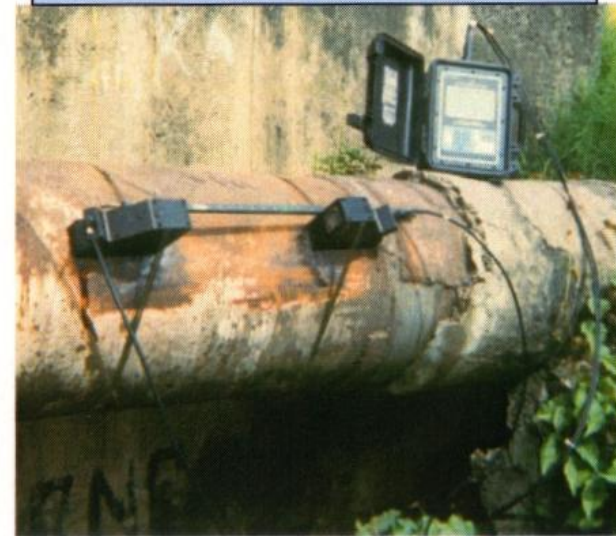
At the distribution pipe
