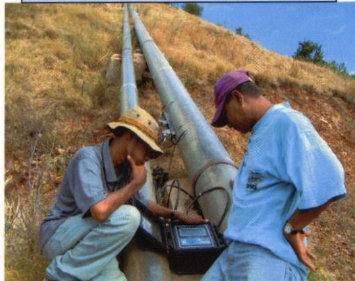
At the distribution mains
