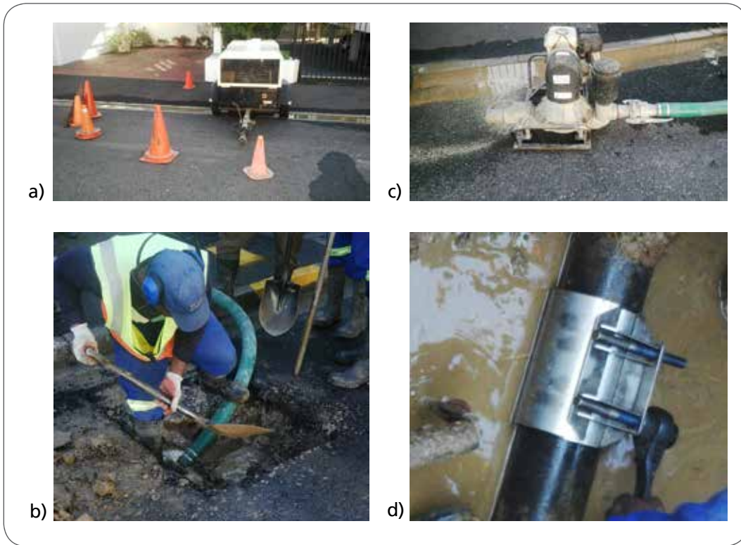
Figure 13 Some steps in the pipe repair process: a) ensuring the work area is safe; b) carefully excavating the pipe; c) draining water from the hole; d) repairing the leak with a repair clamp.
