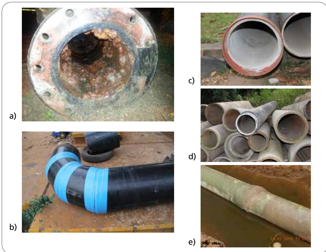
Figure 10 Samples of different pipe materials: a) flanged cast iron pipe showing corrosion tubercles; b) steel pipe with protective wrapping; c) steel pipe with cement mortar lining; d) AC pipes; e) GRP pipe
