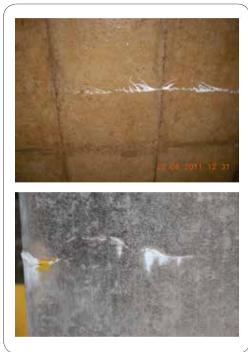
Figure 5 Efflorescence on the outside of a water retaining structure.
