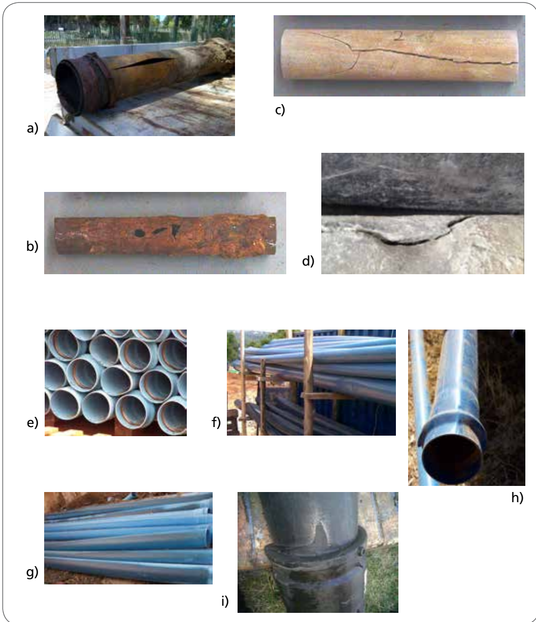
Figure 12 Examples of failed pipes in water distribution systems: a) longitudinal split in a steel pipe; b) corrosion holes in a steel pipe; c) longitudinal crack ending in a bell shape in an AC pipe; d) erosion damage due to soil agitation on the outside of an AC pipe with a longitudinal crack; e) damage due to improper storage of PVC pipes; f) damage due to PVC pipes improperly stored against unprotected wooden poles; g) black discolouring indicating permanent damage to the structure of PVC pipes improperly stored in direct sunlight; h) damage to PVC pipes due to negative pressures; i) poorly done electrofusion weld on an HDPE pipe (note the melted plastic that flowed out of the joint).
