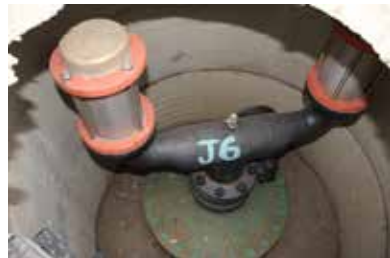
Figure 14 Examples of valves: a) large butterfly valve with a small butterfly valve on a bypass pipe; b) scour valve; c) scour pipe outlet; d) air valves.
