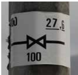
Figure 19 Examples of pipe and valve markers
