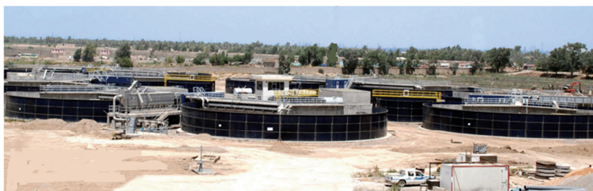
Plate 1 SBR units at Al-Rustamiya WWTP
