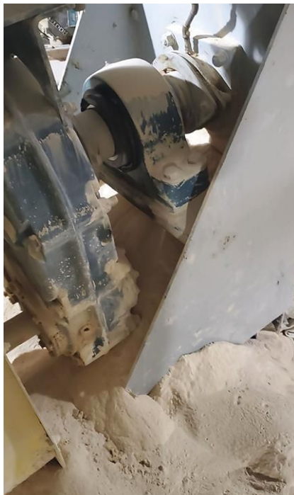
IMAGE 3: Heavy leakage from a screw conveyor moving gypsum
