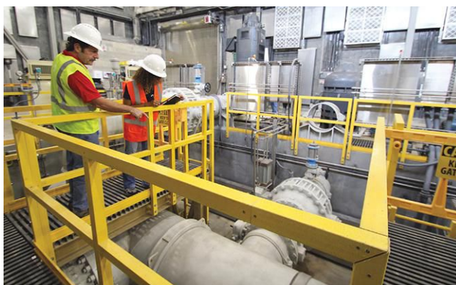
IMAGE 2: Pump discharge piping showing the below grade installation and the pipe support for future above-grade discharge.
