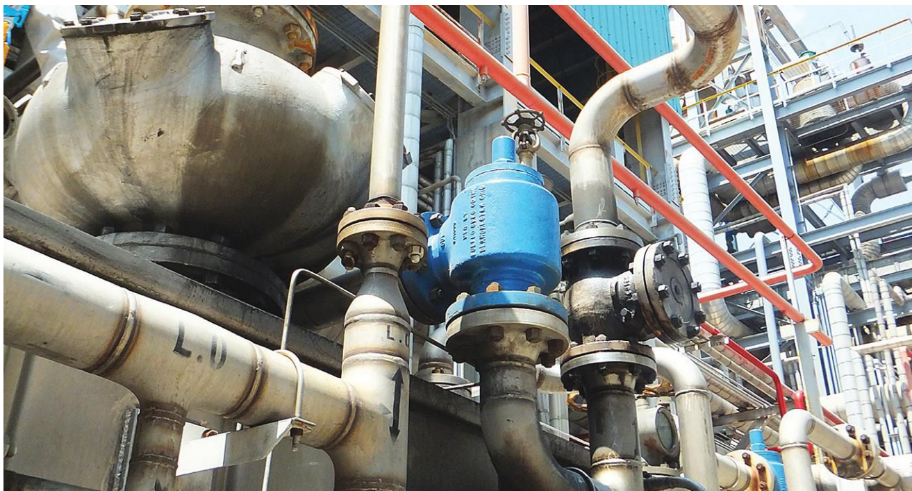
IMAGE 4: A guided piston valve controls line pressure at an oil refinery
