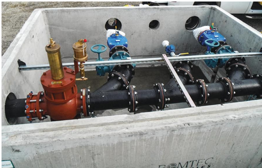
IMAGE 4: Pumping system at Port Arthur, Texas, refinery site
