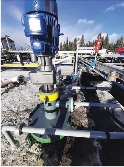
IMAGE 3: Progressive cavity pump installed on top of a knockout drum
