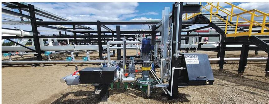
IMAGE 2: Oil and gas facility
