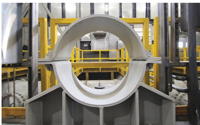
IMAGE 3: Custom-designed carbon steel pipe support for future above-grade pump discharge piping
