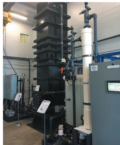
IMAGE 2: Biofiltration column with underdrain
