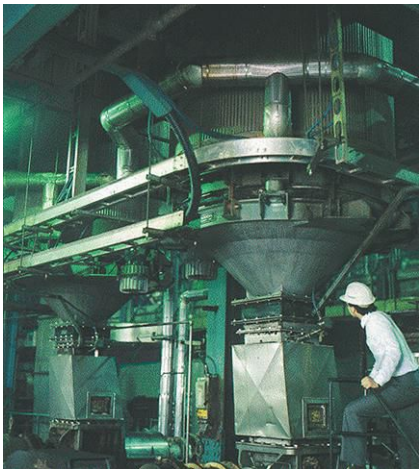
IMAGE 1: Wood chip feeder bin with rectangle expansion joint (Images courtesy of Fluid Sealing Association)
