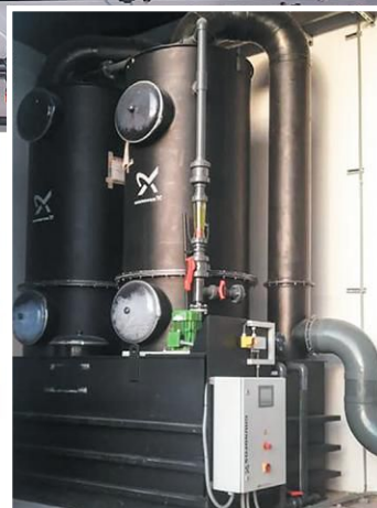
IMAGE 2: Chlorine neutralization system
