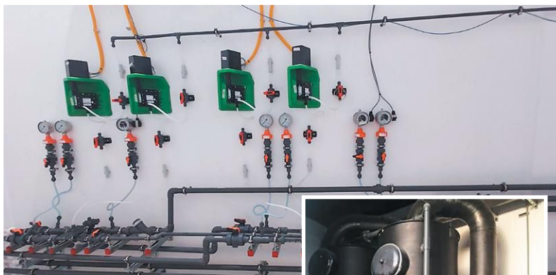
IMAGE 1 (above): Chlorine gas dosing system controlled by a dedicated chlorine gas control panel (Images courtesy of Grundfos)
