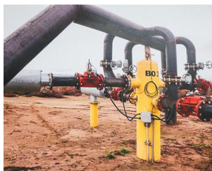
IMAGE 4: A main pipeline connects to a cluster where two to four pivots are fed with a tank head. The pivot pipes leave this location and go out to the center pivot. These clusters contain all electrical, control wires, water valves and cluster pressures. This is where the pivot control panels are located along with network communications equipment.
