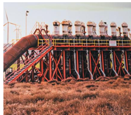
IMAGE 3: The pump stations were retrofit with upgraded programmable logic controllers and fitted with medium-voltage VFDs to control the motor/pump speeds to anything between zero and 100%.
