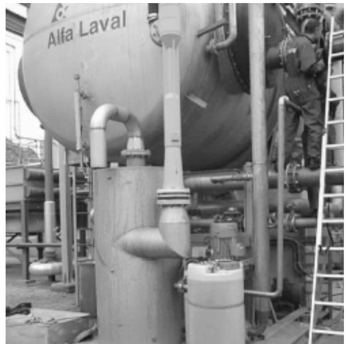
Fig. 73: MED distillation system with dosing unit for anti-scaling agent (front right)
