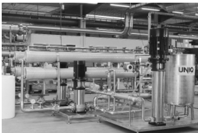
Fig. 53: Membrane system for filtration of brewery wastewater including two dosing systems
