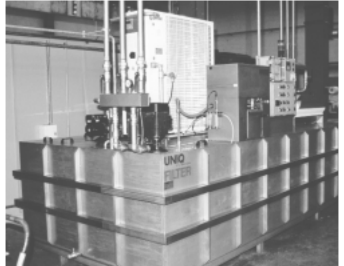
Fig. 26: Central system with two bands, holding tank, cooling system and pumps
