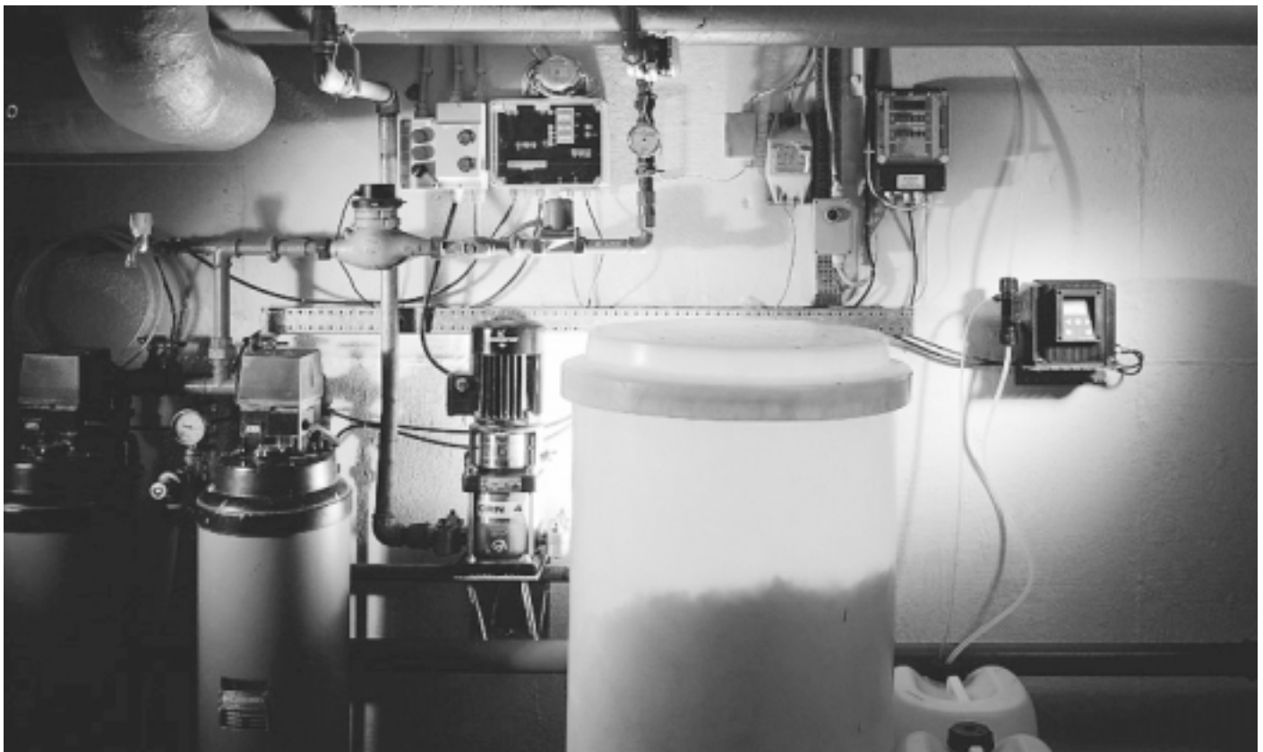
Fig. 77: Dosing of base for pH control of the water in district heating system and boiler
