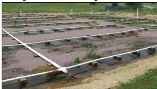
Neglected Recirculating Media Filter
