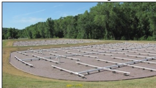
Well-Maintained Recirculating Media Filter
