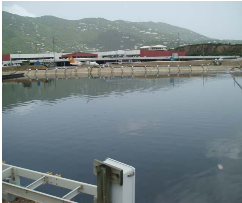
Figure 3.4 The Middle Basin of the Airport Lagoon Treatment Plant Located Southwest of the Cyril E. King Airport
