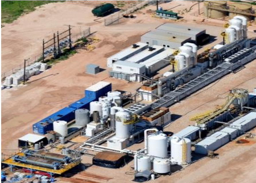
Carrier gas extraction plant using HDH technique
