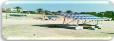
PV testing units
