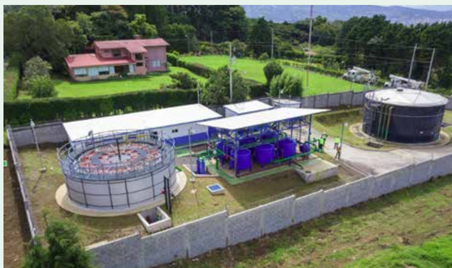
Figure 6. Full view of Breña Mora PWTP - Radial flow settlers with SDM (source: LE)
