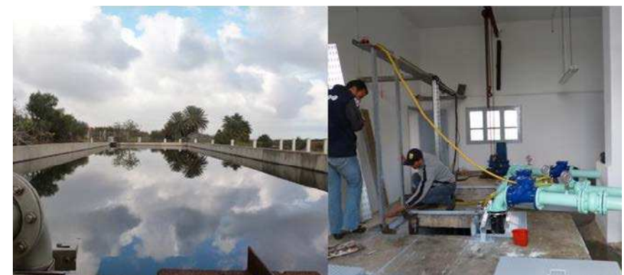
Figure 6: Storage basin of 1,000 m 3 and maintenance of the pumping station in Ouardanine (with permission of O. Mahjoub 2015)
