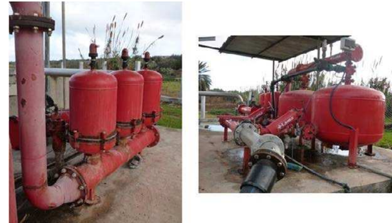
Figure 8: Battery of filters at the outlet of the storage basin (with permission of O. Mahjoub 2015)
