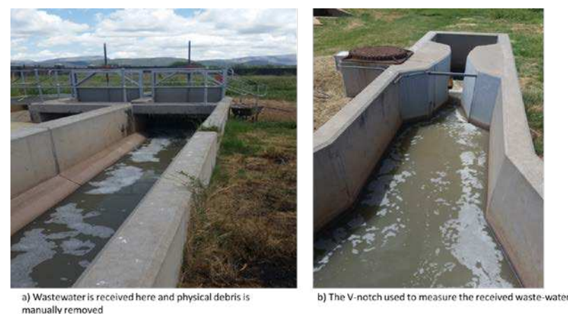
Figure 2: Physical screening of solid waste and V-notch weir at Lebowakgomo wastewater treatment plant
