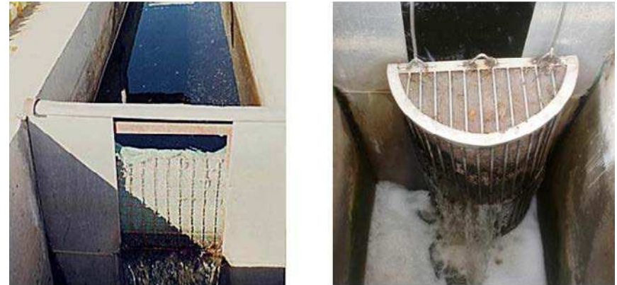
Figure 7: Net installed at the outlet of the WWTP in Ouardanine in 2003 (left) and the new sieve and net installed in 2004 (right) (with permission of O. Mahjoub, 2003, 2015)
