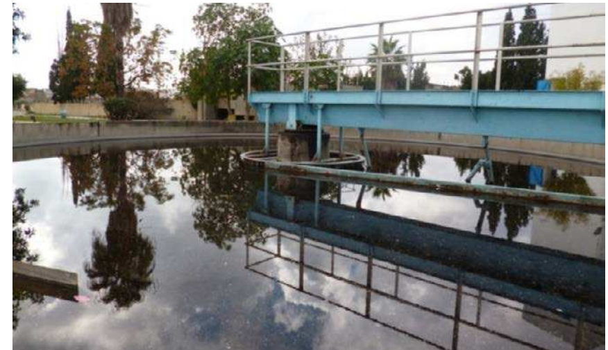
Figure 3: Secondary clarifier at the WWTP Ouardanine (with permission of O. Mahjoub 2015)
