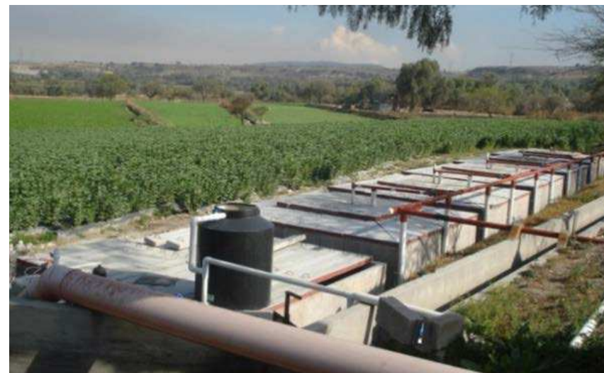
Figure 2: WWTP with quinoa crop (Acoculco, Hgo.)
