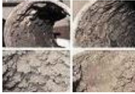
Fig.5.4: Scales Formed Due to Corrosion
