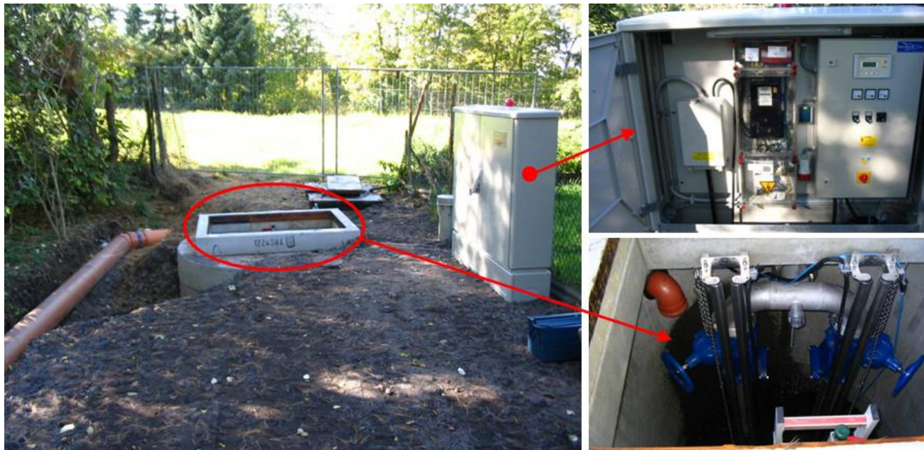
A sewer pumping station in Germany with the pump shaft and the electricity/control unit.
