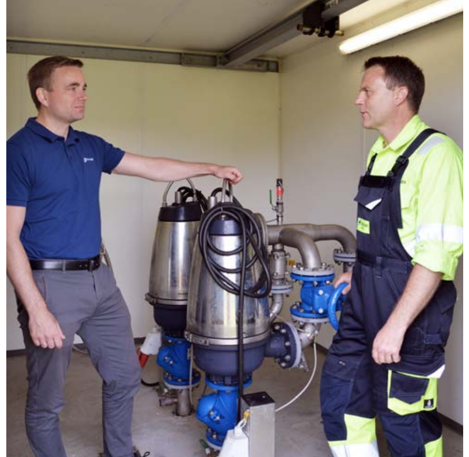
Operations manager Casper Nordow Koch, Provas, is excited about the prospect of transforming real time sewer network data into actionable information and ultimately optimize the efficiency the sewerage system.
