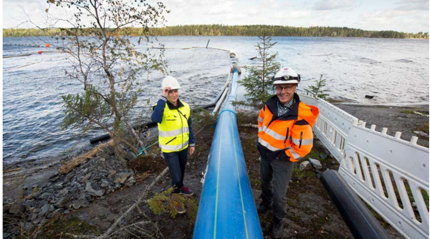
The water supply system in the city of Tampere covers a network of approximately 780 km. New underwater mains pictured waiting for submersion.
