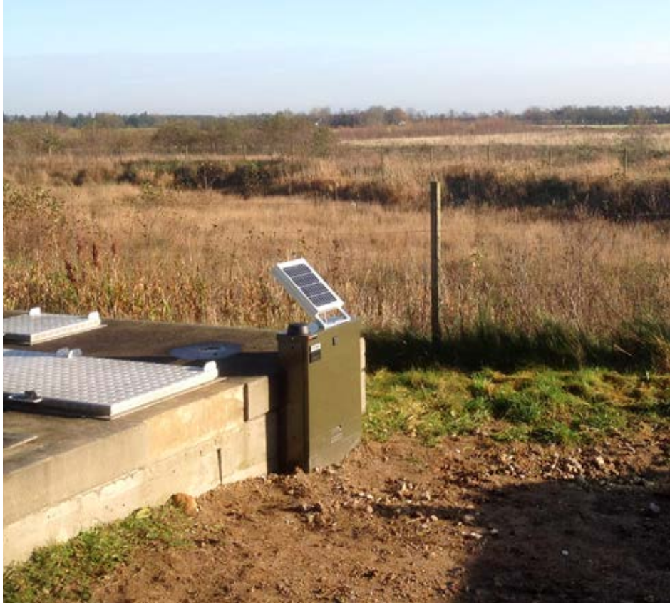
As sewer overflows are often very remote, and rarely established with a main power source – the complete system is battery powered, with the possibility of direct connection to a small solar panel, for permanent operation.
