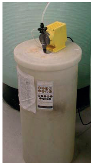
Picture: Sodium Hypochlorite Tank and Hypochlorinator
