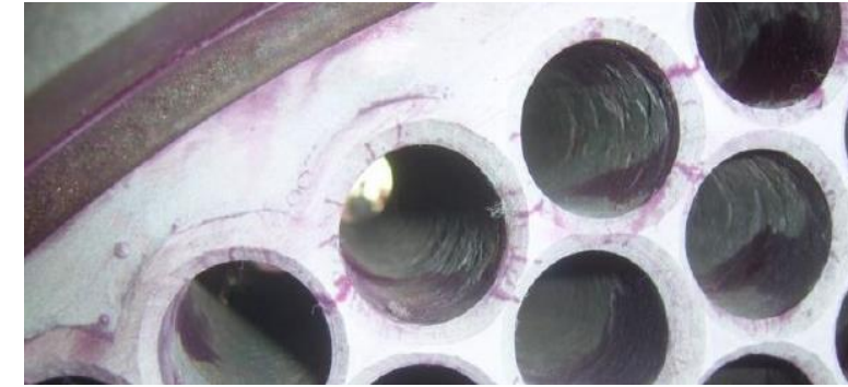
Multiple Cracks in TTS as detected by DPT
