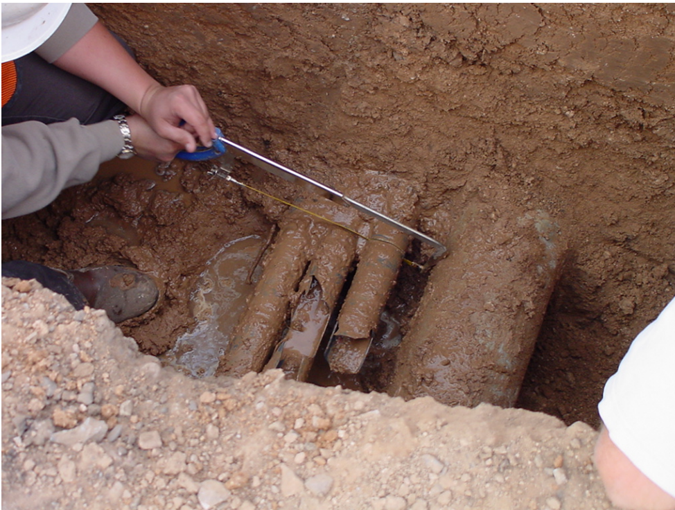
Service worker cutting abandoned utility conduit out of the way. Always call first and get the utility to show up to verify if you are able to cut an abandoned utility. I personally do not trust anything the other utilities will say or put in writing.
