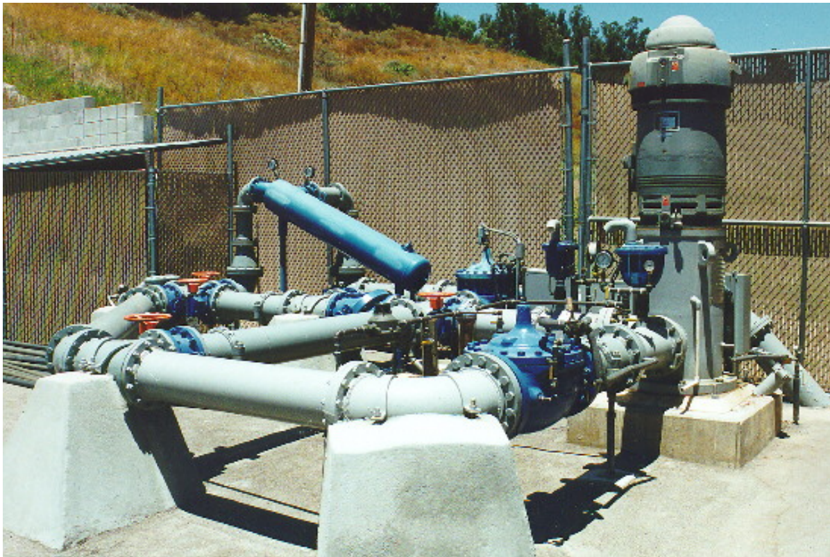
Vertical Turbine Well
