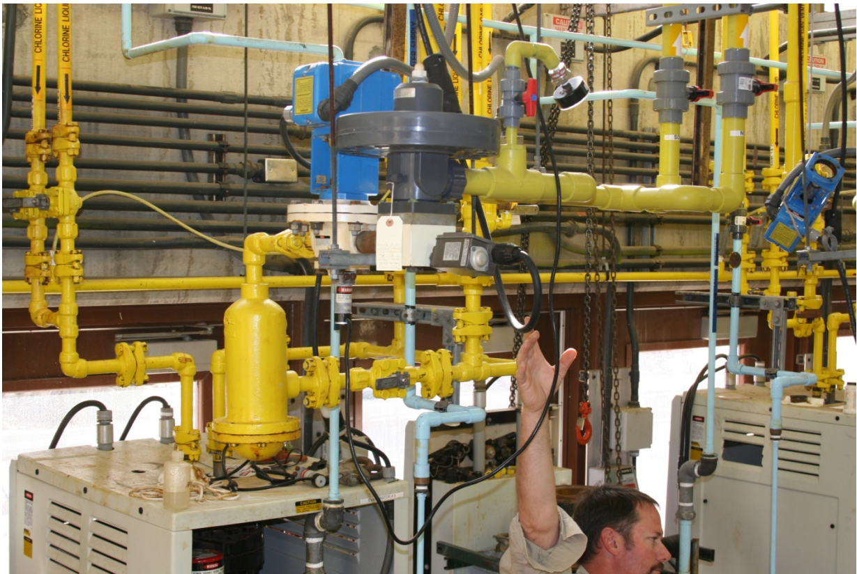
Chlorine gas piping.
