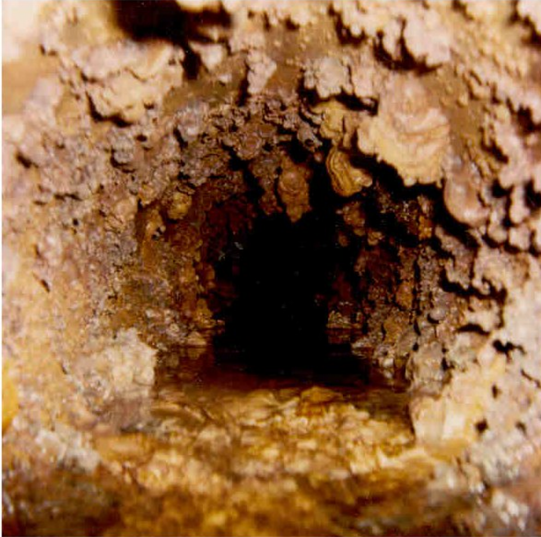
Notice the corrosion inside this cast iron main.
