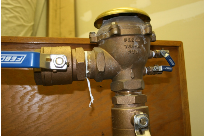
PRESSURE VACUUM BREAKER ASSEMBLY
