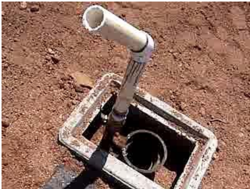
A temporary blow-off at a dead-end line.
