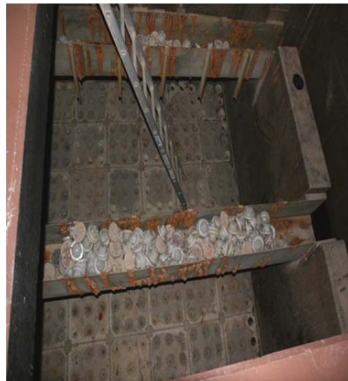
The photograph on the right shows a filter support bed under construction.
