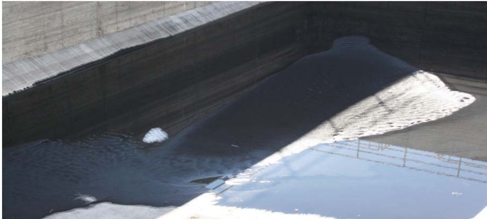
A photograph of a backwash basin that has media caked on the bottom.
