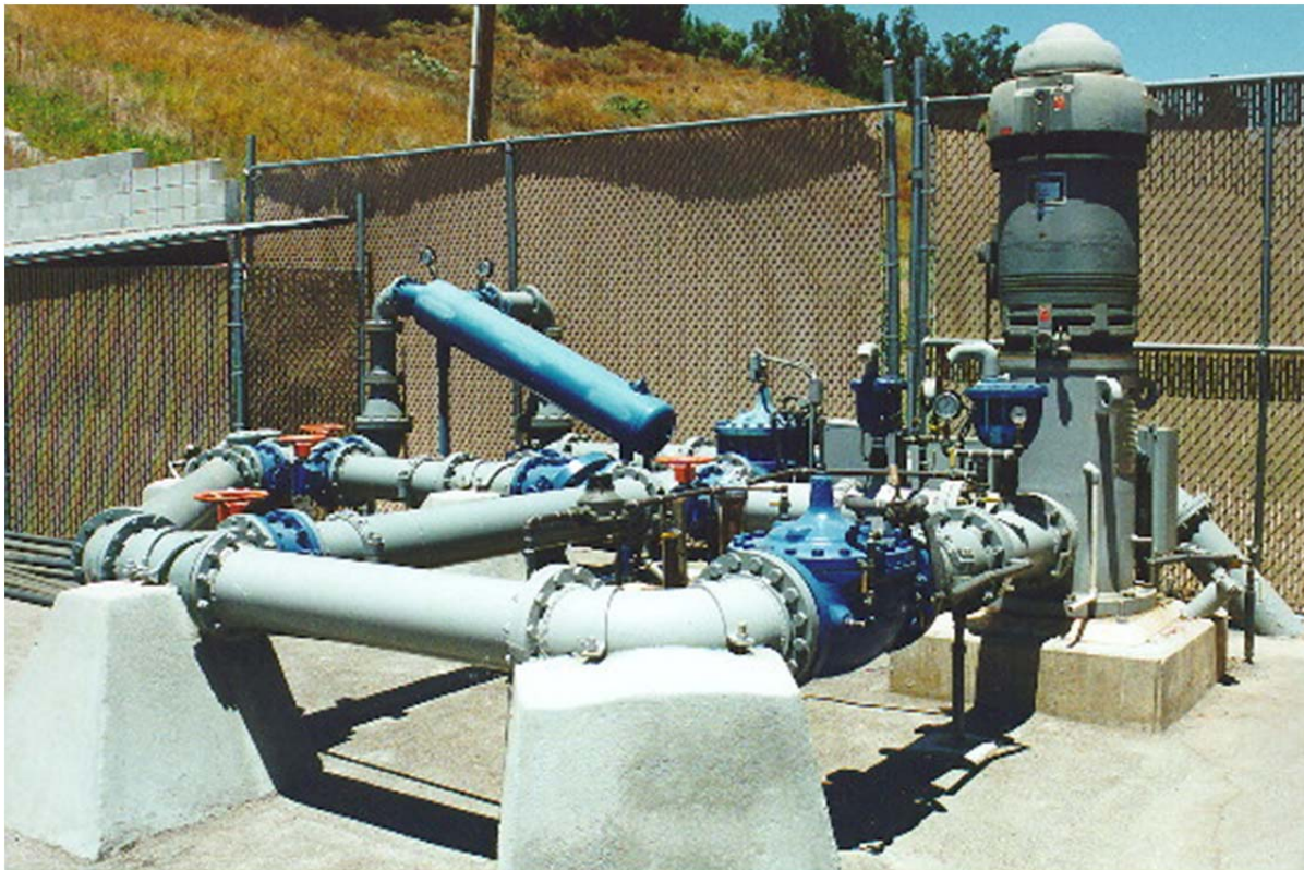
Vertical Turbine Well
