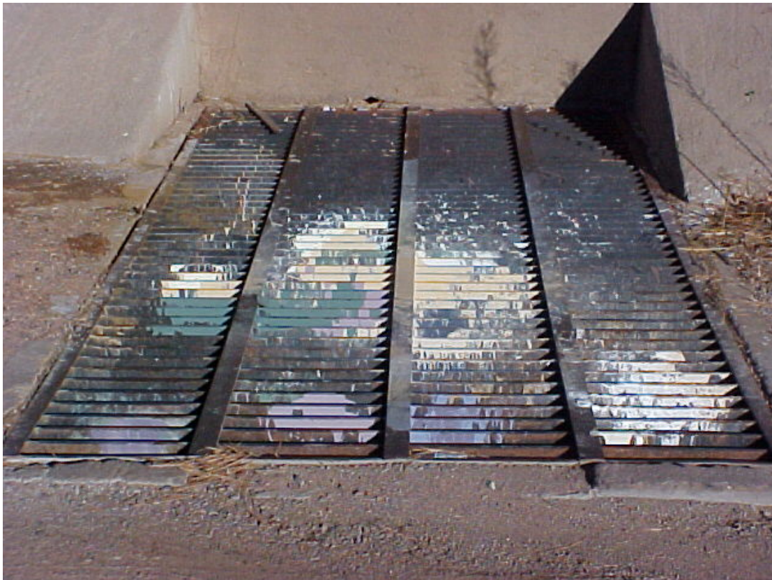
Evidence of illegal paint and chemical dumping.
