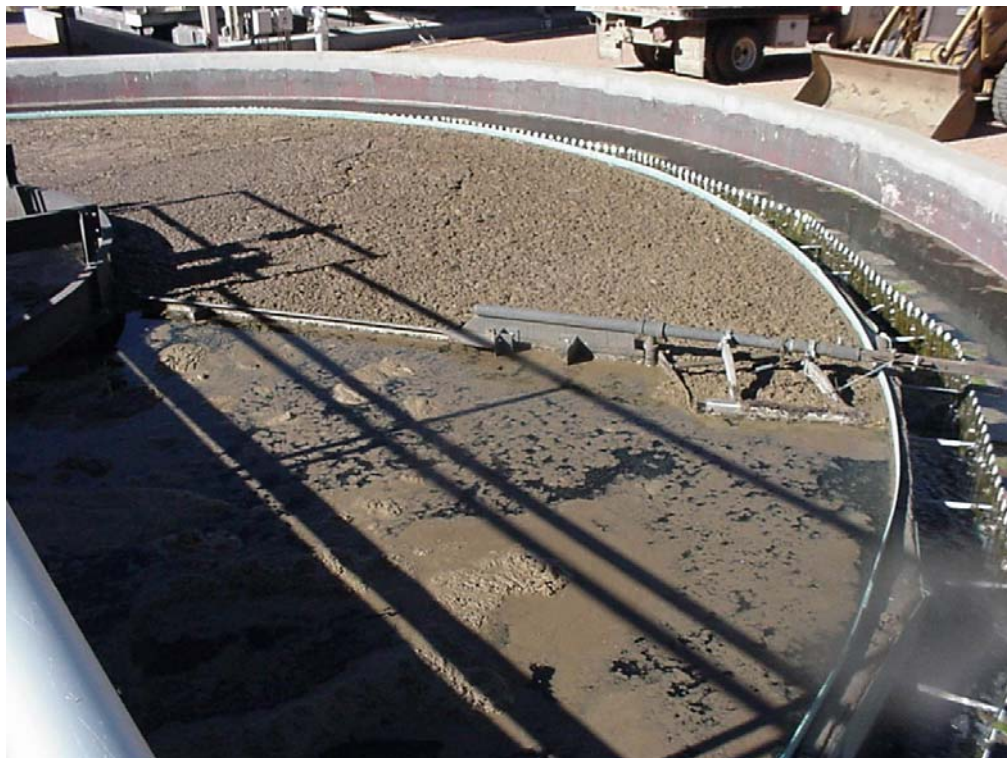
Primary Wastewater Treatment Clarifier.
