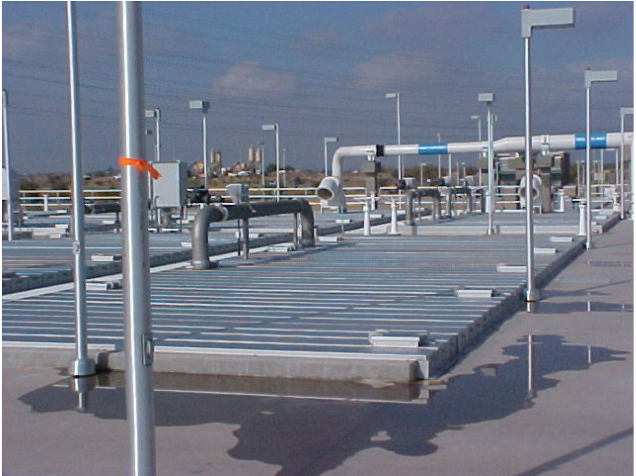
Covered basin used for odor control
